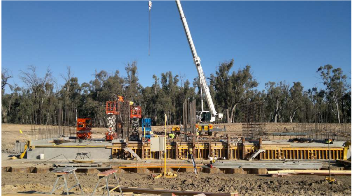
Construction works at Calf Creek regulator site. Photo courtesy of Lu Rathje from Professional Engineering Services.
