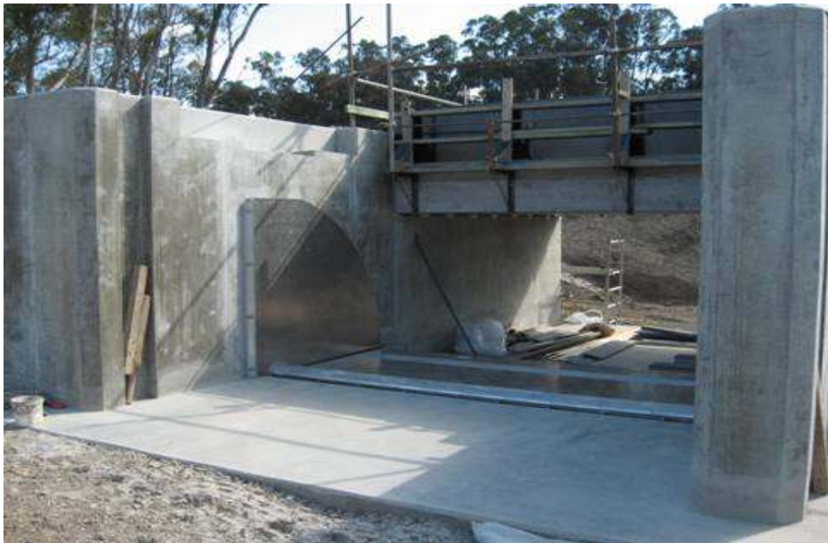
Tilt gate installed at the Return Channel regulator. Photo courtesy of Professional Engineering Services.
