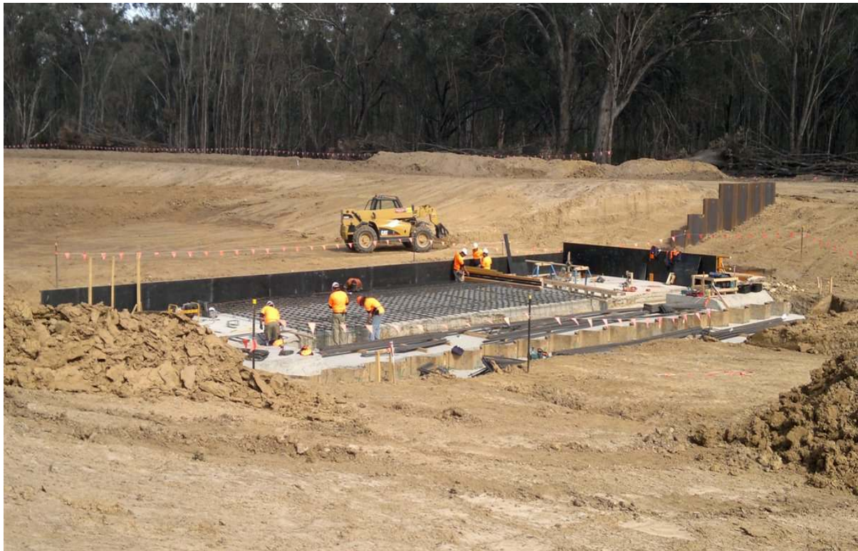
Foundation works and preparation for concrete pouring at the Inlet Channel regulator work site. Photo courtesy of Peter Arnold from Professional Engineering Services.
