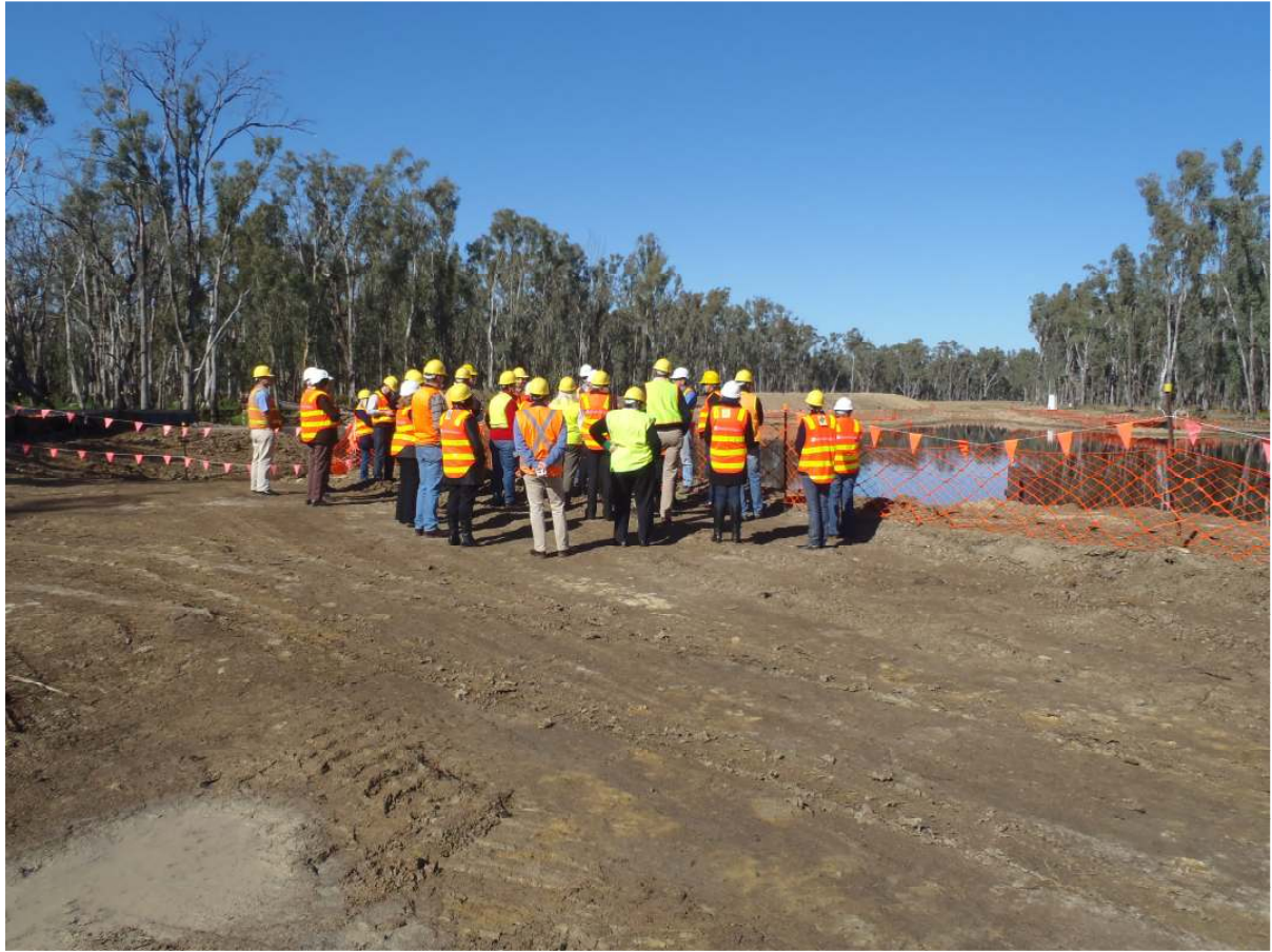
Delegates from the Rice Growers Association inspecting the Barber Creek regulator work site and levee works.
