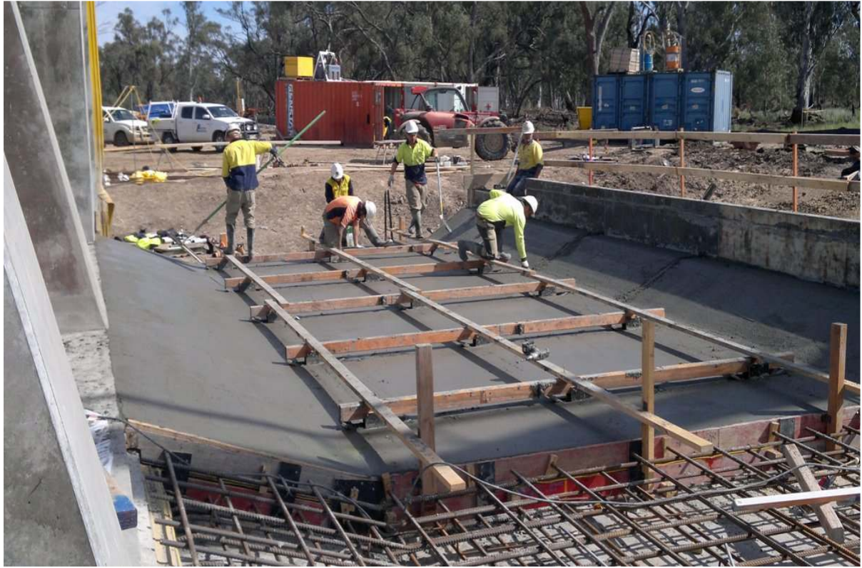
Concrete work as part of the Calf Creek regulator downstream apron. Photo courtesy of Professional Engineering Services.
