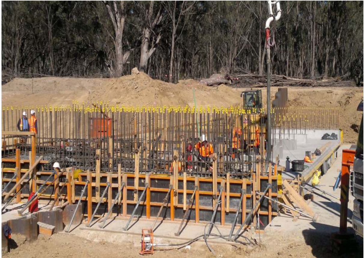
Pouring of concrete for the floor slab section as part of the fishway entrance on the inlet regulator structure. Photo courtesy of Professional Engineering Services.
